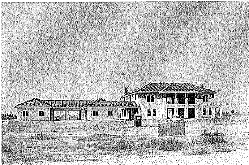
New Home being built on South "H" Street northwest of the Bakersfield College South Center Campus Site.
